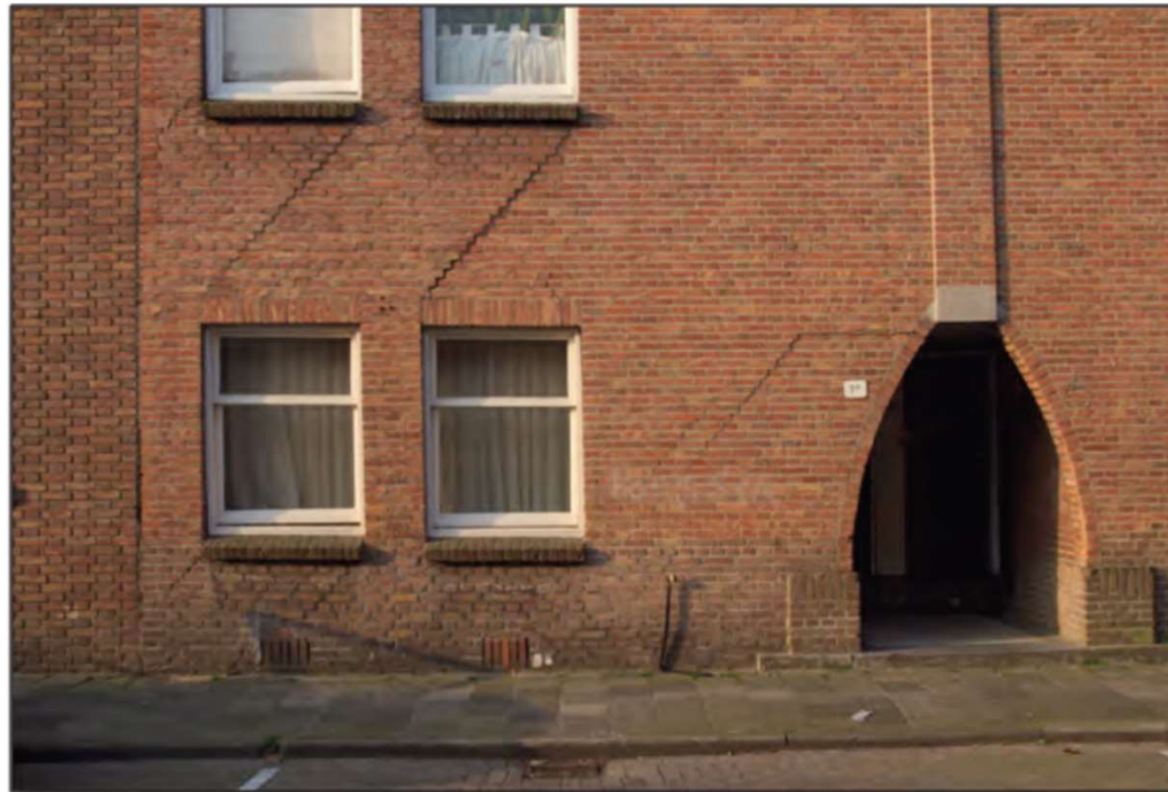
Fig 1.3.1e Various parallel cracks from bottom-right to top-left in wall due to rotting foundation piles. Source: Peter Dorsman
